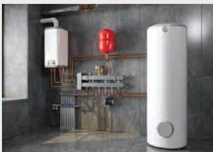
GAS WATER HEATERS
